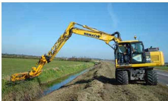
An excavator with the mowing bucket on an extension piece for extra reach.
